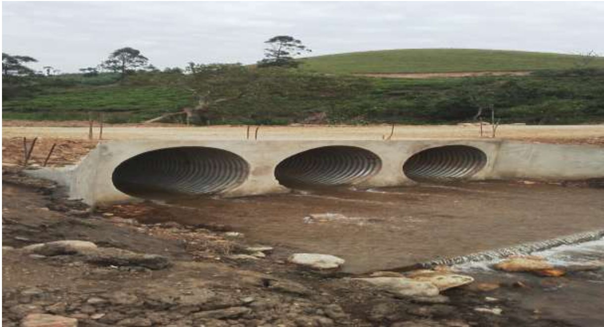
A section of the road in Bitooma repaired under CAIP that was hitherto impassable
