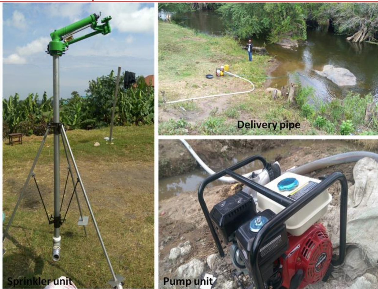
Figure 5-25 Rain gun movable sprinkler irrigation system
