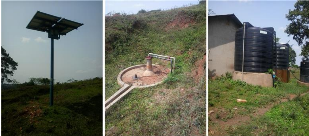
Figure 5-13 A solar powered abstraction adapted on a borehole
