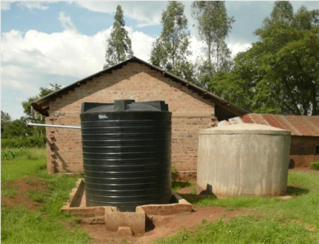
Figure 5-8 Aboveground tanks: plastic tanks (left); ferro cement tanks (right)
